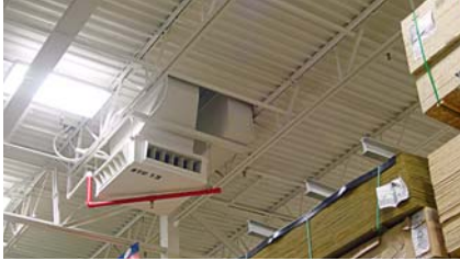
At Lowe's, an existing concentric curb air distribution plenum is now served by the desiccant dehumidification/air conditioning unit.
