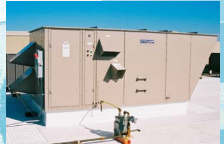
A SEMCO Revolution® natural gas-fired hybrid cooling/dehumidification system supplies moisture-controlled fresh air at a Georgia school.
