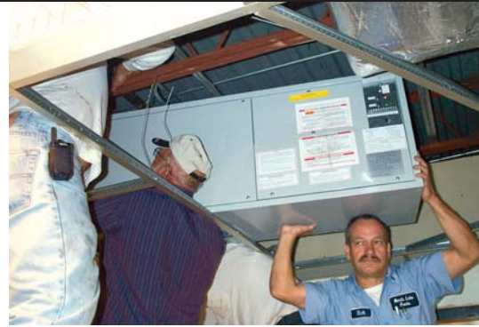
Technicians install a NovelAire® compact desiccant-based dehumidifier under the ceiling tiles at a restaurant.
